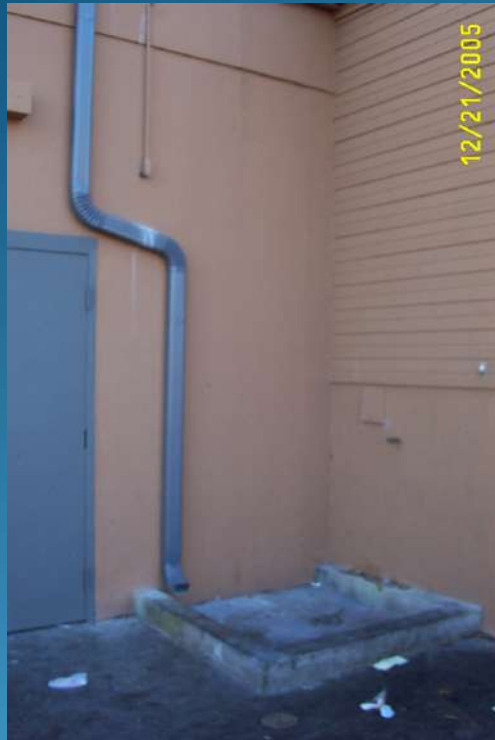
Gutter discharging to mop sink: Inflow & Infiltration
